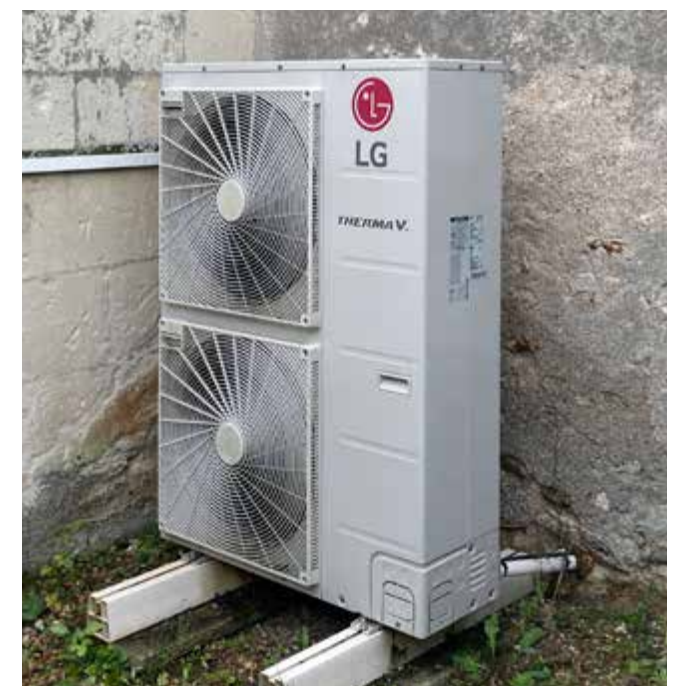
Example of a heat pump installation.
