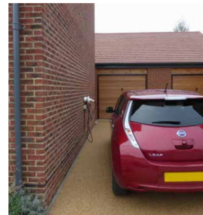
Home electric vehicle charging
